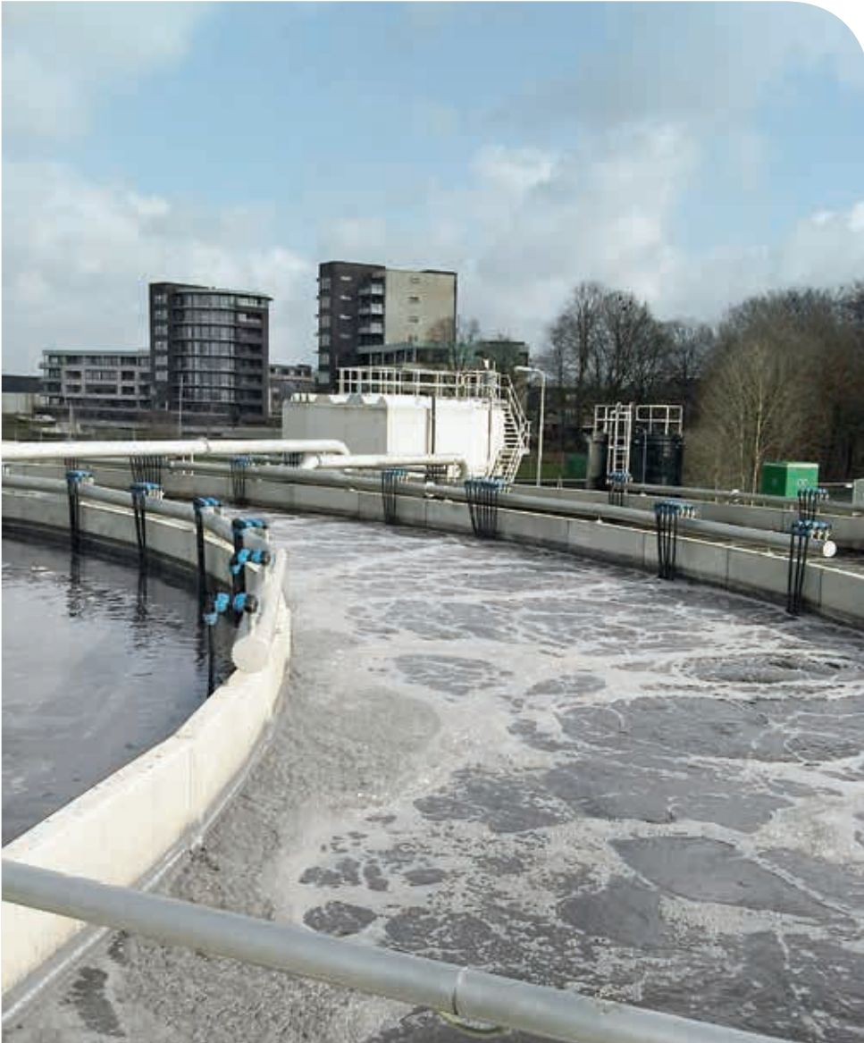
Wastewater treatment plant Steenwijk, Netherlands
